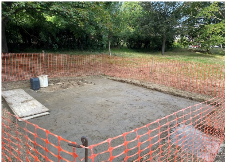
The work that has started on the new picnic area in West Wood.
